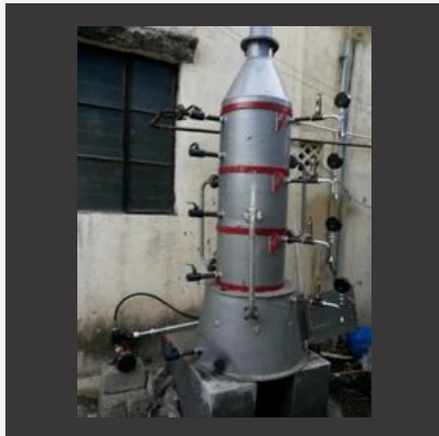
Gas Fired Steam Boiler
